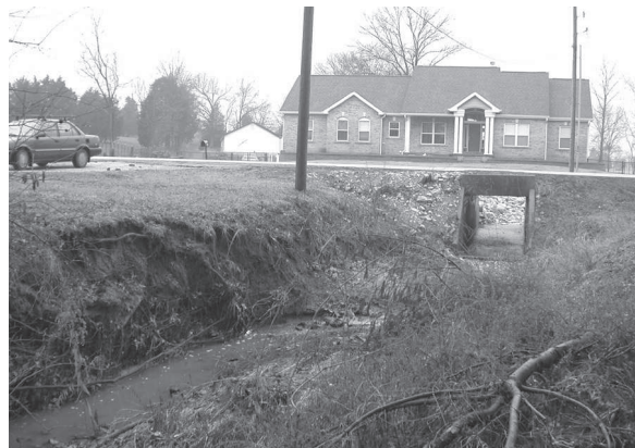
Eroding creek bank.
